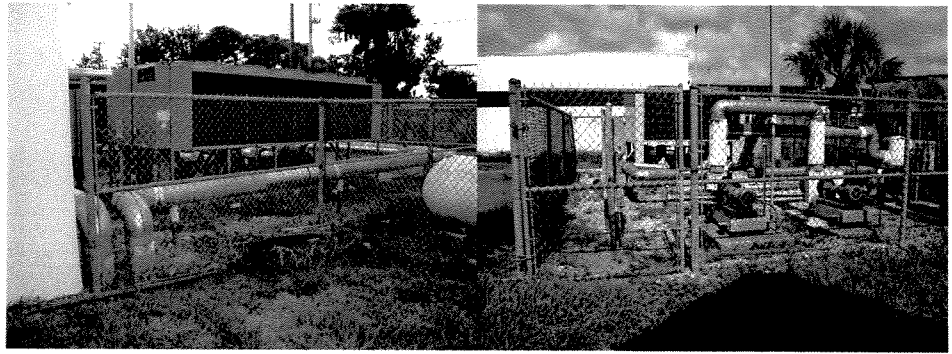
Large chiller plant: CH-1, CH-2
