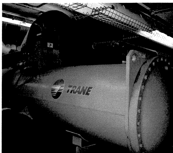
Trane Chiller at Northeast High
